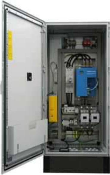
Fig. 12-4 Control cabinet with electrode holder changeover
