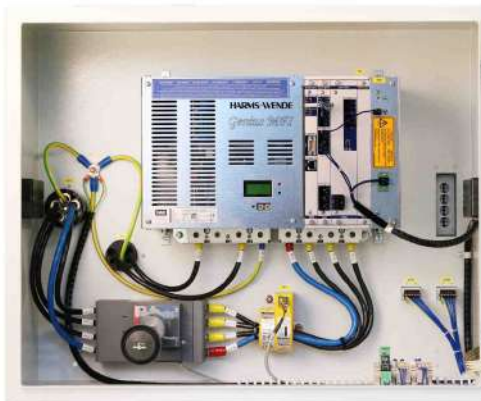
Fig. 12-2 Top mounted robot cabinet, interior view
