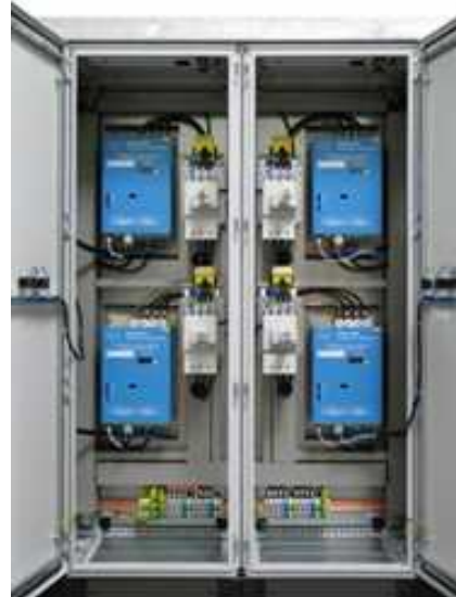
Fig. 12-5 Control cabinet with four inverters
