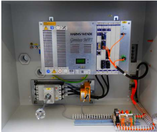
Fig. 5-2 Top mounted robot cabinet, interior view
