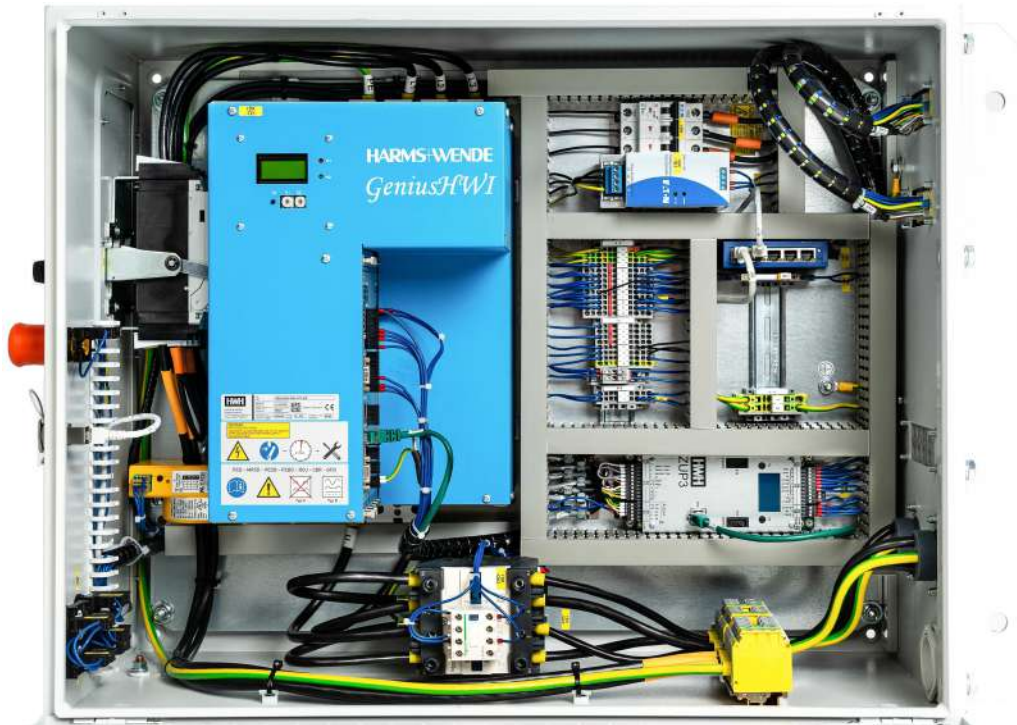
Fig. 5-7 One cabinet with a central switching PCB
