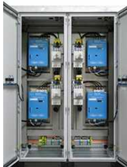
Fig. 5-10 Control cabinet with four inverters
