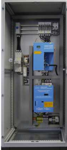
Fig. 5-9 Control cabinet with master/slave
